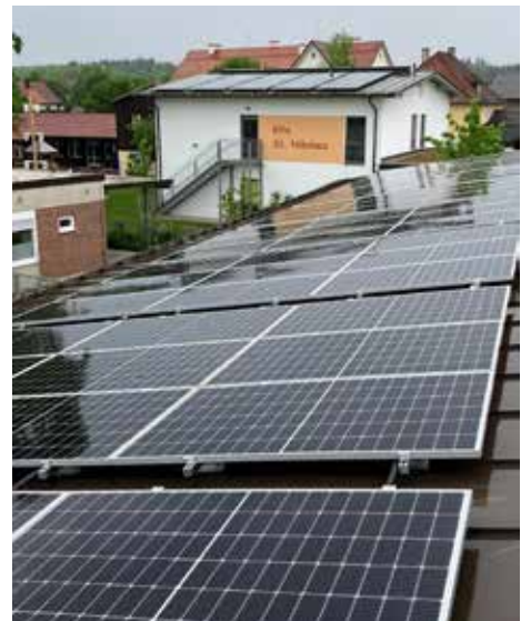
▲ PV-Dachanlage Kindergarten St. Nikolaus in Emmerting.
